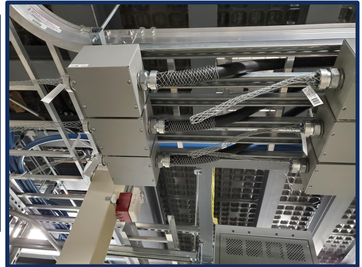
Pre-located J-boxes for HPC Rack Power Whips
