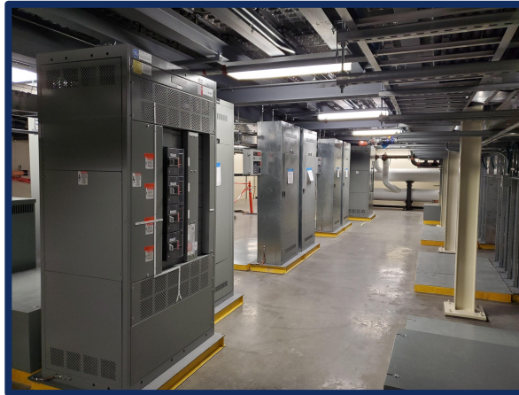
480v Distribution and Branch Circuit Panels - Derecho Compute
